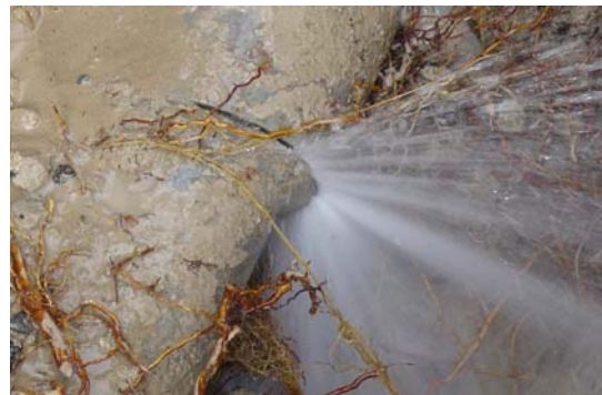
A leaking pipe joint
