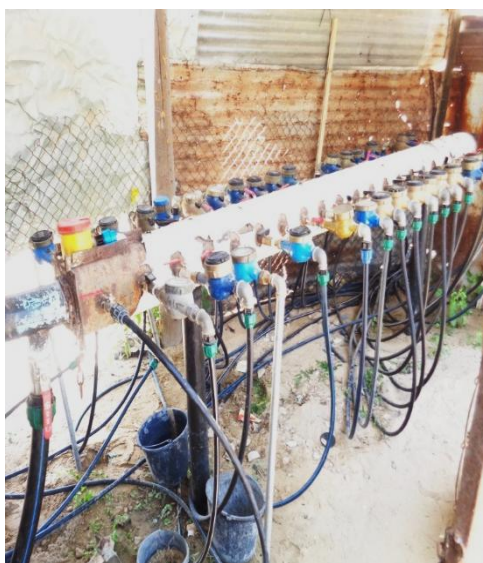
Figure 5. One of the installed central water dispensing units
